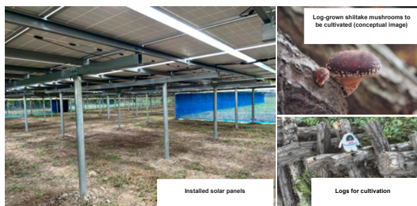
Off-site physical PPA (IKO Agri-Solar, shiitake)
